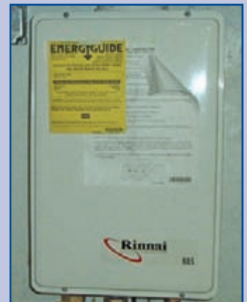
High efficiency water heaters save heating energy, while still providing ample amounts of hot water.
