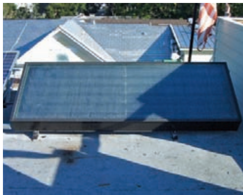
A solar thermal hot water system preheats incoming water.
