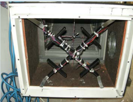
Figure 1. Temperature, humidity, and air flow instrumentation at entry to AHU monitors system operation in real time.
