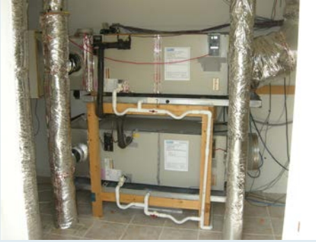
Figure 2. AHUs for SEER 13 (top) and SEER 22 (bottom) 2-ton heat pumps can be connected to indoor or attic ducts.
