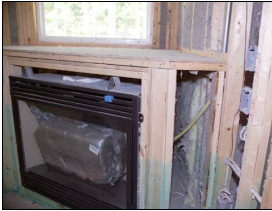
Figure 19 Note that wall behind fireplace is insulated as required by the TBIC.
