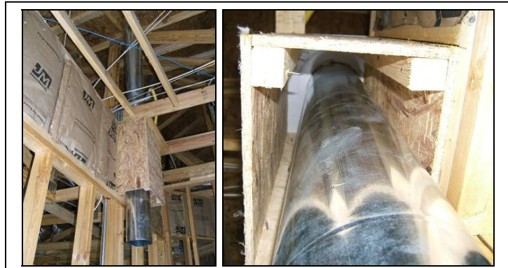
Figure 10 Chase (l) for kitchen exhaust fan duct. Top of chase (r) is sealed to reduce infiltration.
