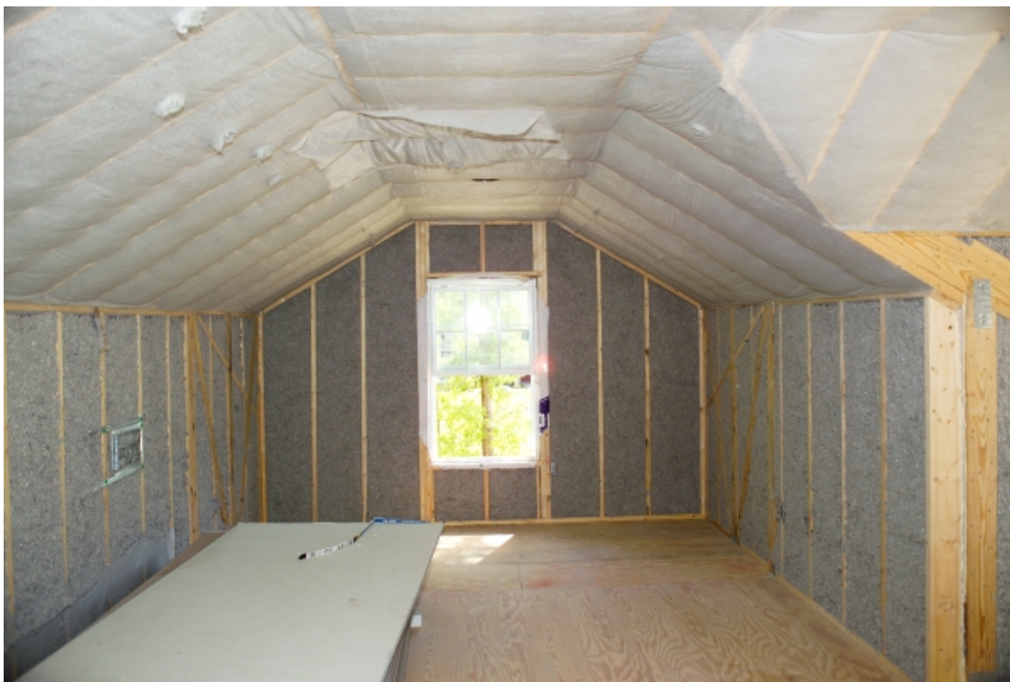
Figure 21 Inspection of the R-13 cellulose in G. W. Robinson Builders' home to verify it has been installed with no gaps, compression, or voids as required by the TBIC.
