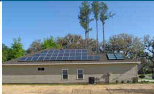
6.6kW p photovoltaic system and 120 gallon solar hot water system
