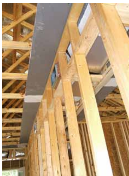
Ducts within conditioned space with custom short boots
